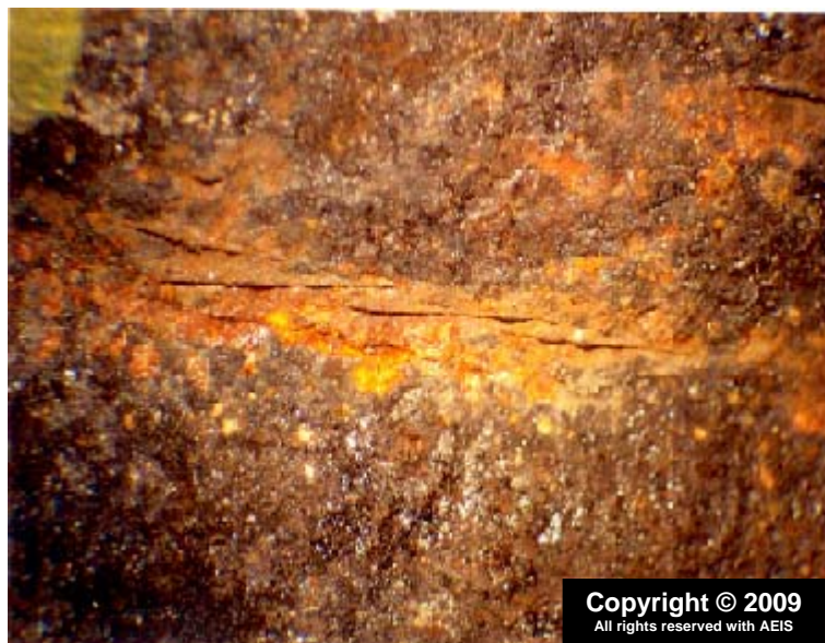
Figure 5: Outside Surface Mechanical Dent Marks in the Weld Zone
