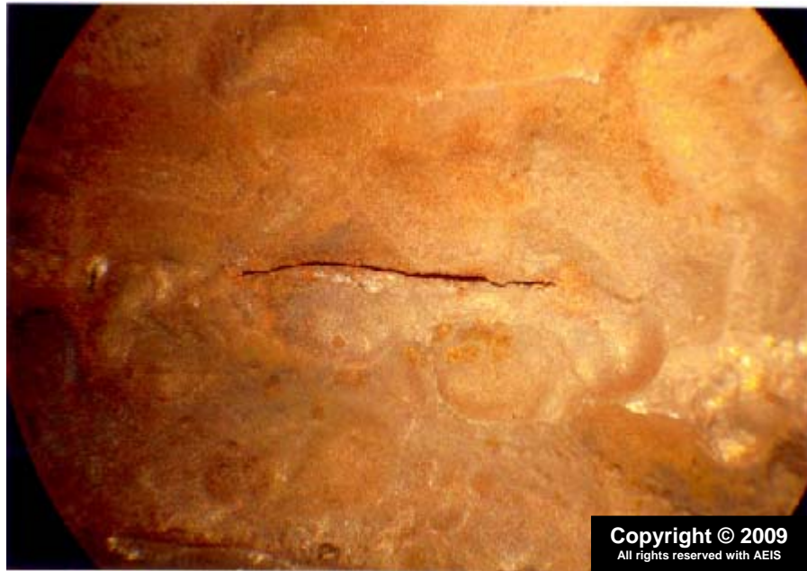
Figure 3: Crack Lips on the Inside Surface
